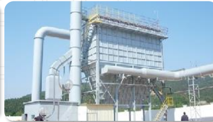
Waste Gas Treatment
