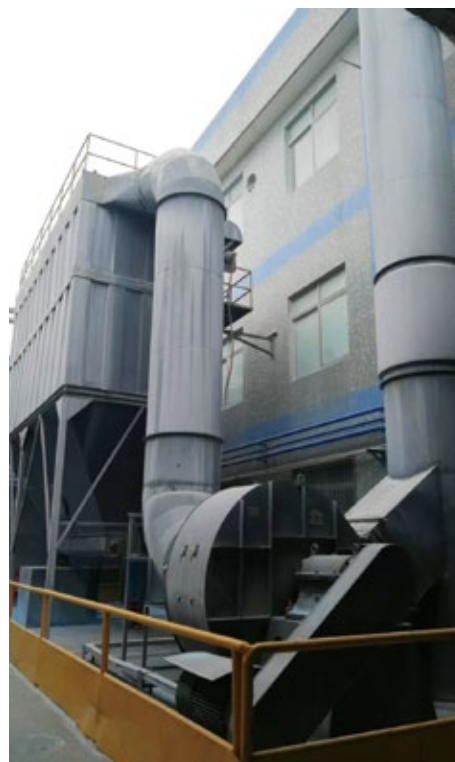
Workshop Dedusting Equipment 車間除塵設備
