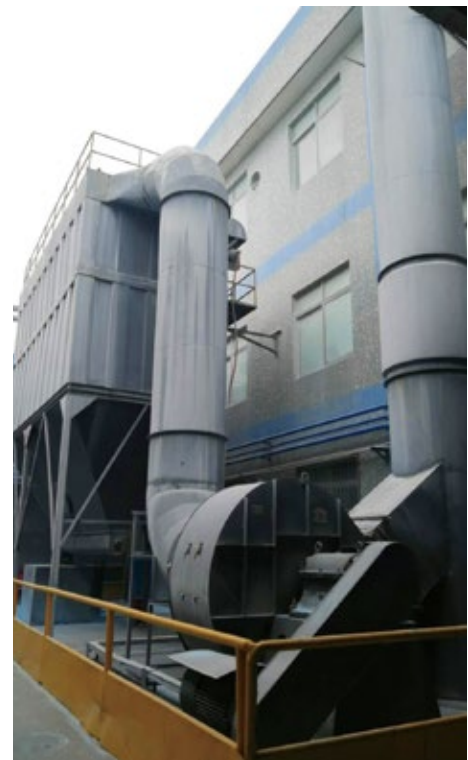
Workshop Dedusting Equipment 車間除塵設備
